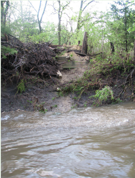
Damaged east support structure
